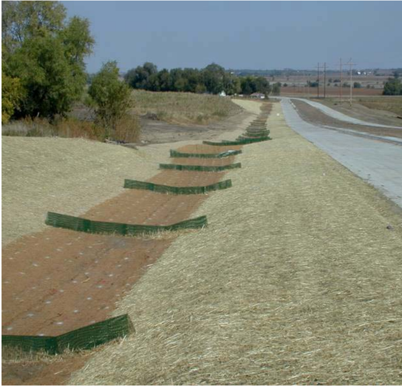
Proper road ditch and shoulder stabilization using erosion control blankets in the watercourse, Georidges and mulching. (Photo courtesy of Fred Kelley.)
